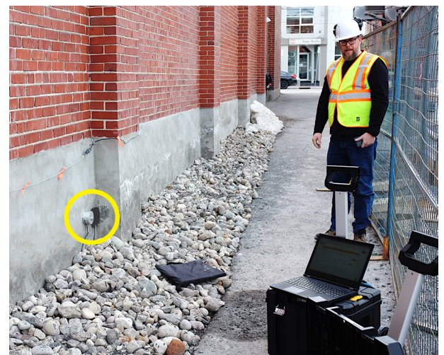
Figure 26. The MEMS and solenoid devices were mounted side-by-side along a concrete wall on an adjacent building to the construction site, 18 inches above the ground.
