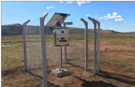
Vibration Monitor Housing and Relay Station
